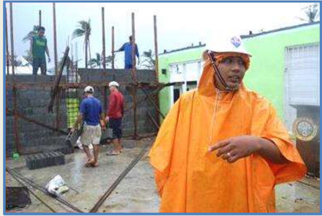
AMURT Engineer 'Boy' supervises school repairs at Central Elementary School in Mercedes Municipality
