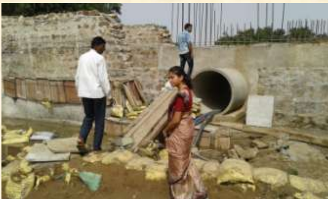
Check Dam near AMIT / Baba's Memorial
