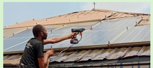
Five of the AMURT assisted health center now have solar power. Cleaning the panels in the dry season is an important part of maintenance.
