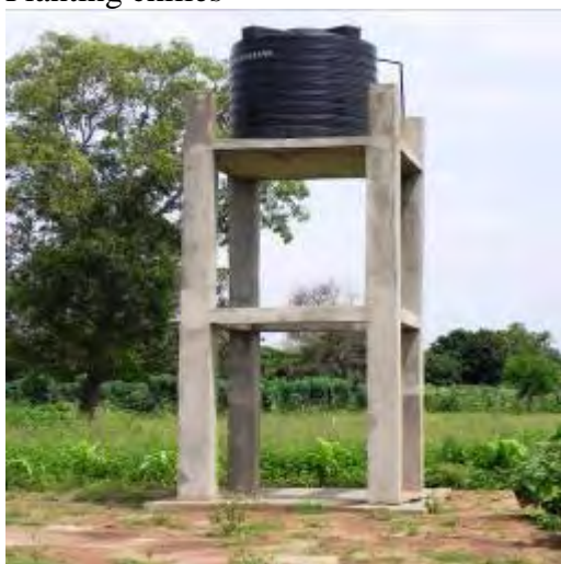
The tank on the bore hole
