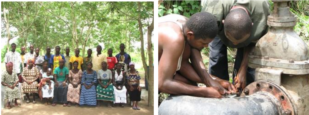
Left: Headmen and standpipe attendants at Southern Zone monthly meeting in May; Right: Omoro and Moses installs the new big wall to control overflow on the dam
