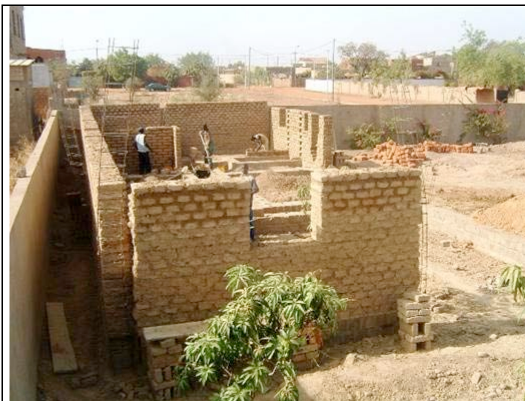
Construction underway on the new jagrti and AMURT center in Ouagadougou. Supervised by b traditional local materials. It will be an ecological building.
